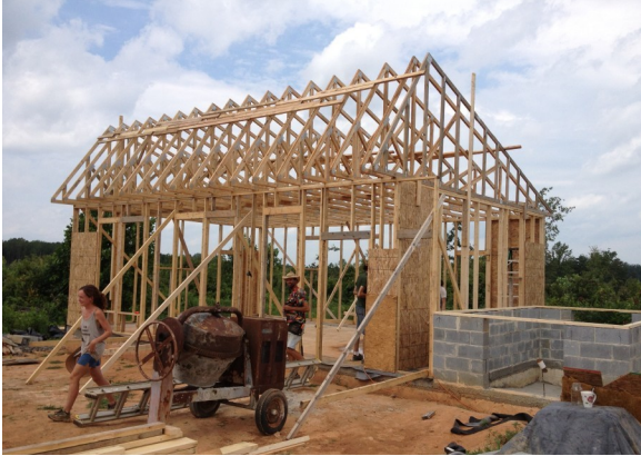
Kitchen skeleton: the entire south-facing roof will be a solar collector
