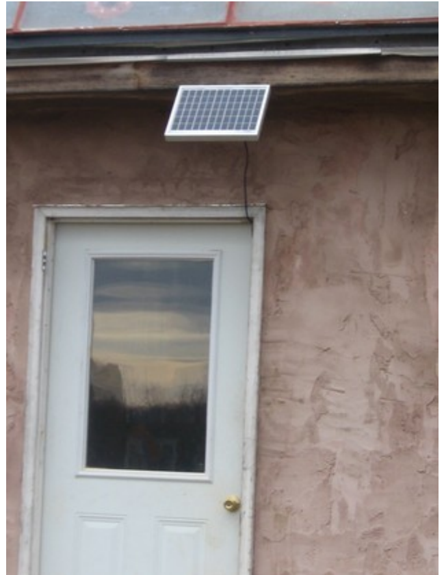
LELS systems are extremely efficient. One 10 watt solar panel is enough to keep the lights on in a small house.
