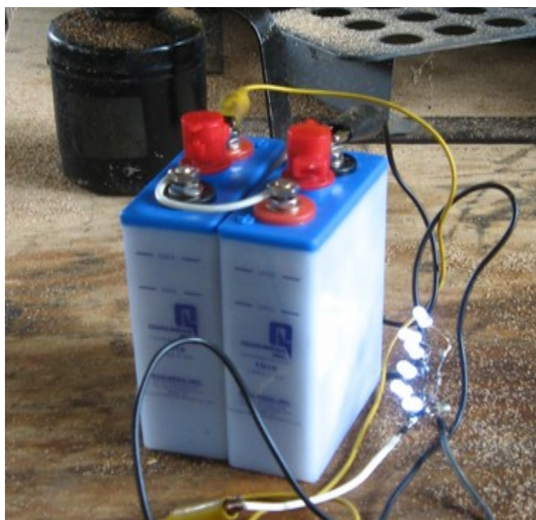
Two cell NiFe set, $36 in batteries, 6 cents in LEDs, no charge or discharge regulation necessary. The "bulb" here has been burning for over a week.
